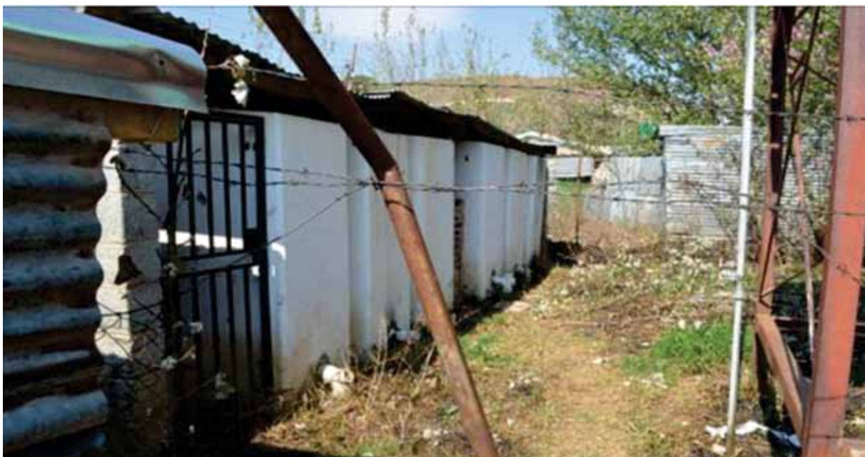
Toilets at the bus shelter and around are currently not functioning and are locked.
